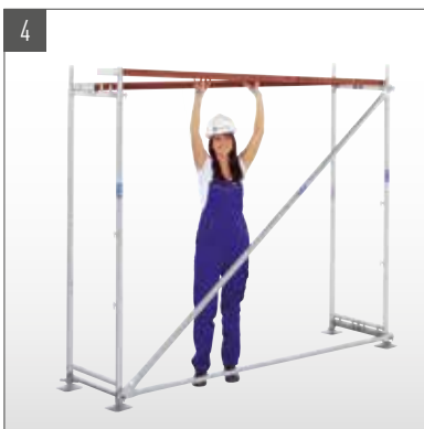
Mount decks, align scaffold bay perpendicularly to guard rail and frame using spirit level.
